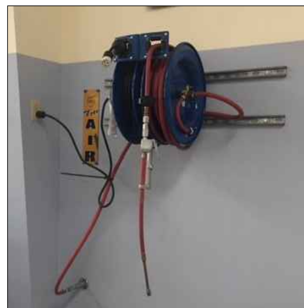
Wall Mtd Air Reel 2 Not to Scale WALL MOUNTED AIR REEL W/ CONVENIENCE OUTLET CONNECTED TO SERVICE BAY AIR COMPRESSOR
