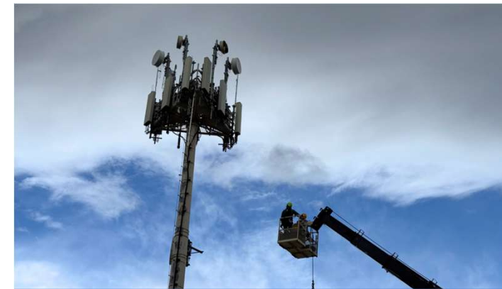
New wildfire camera installed in Minden
